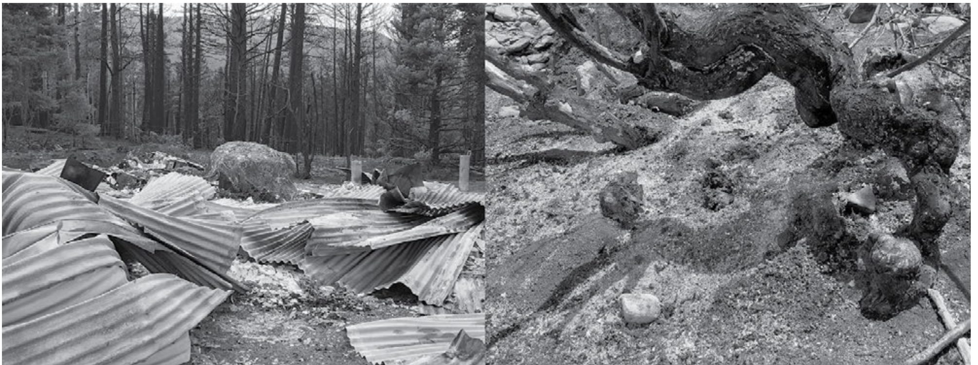
ABOVE: ACEQUIAS: DAMAGED HEAD GATES FROM POST HERMIT'S PEAK + CALF CANYON FIRE FLOODING. ACEQUIA DE LAS COLONIAS, CHACÓN, NEW MEXICO AND ACEQUIAS ENCINAL AND CAÑONCITO, HOLMAN, NEW MEXICO
